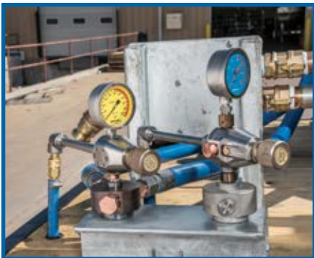
Dual Pressure Control Station
